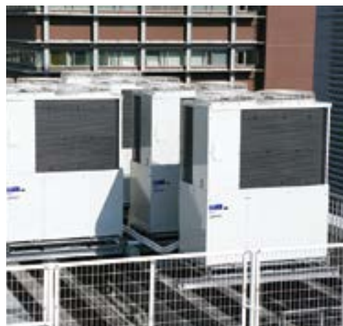
GHP (Gas heat pump air conditioning system)
