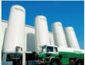
High-pressure gas supply facilities
