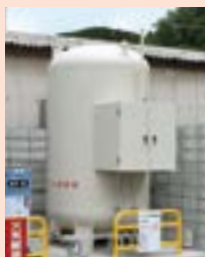
LPG supply equipment
